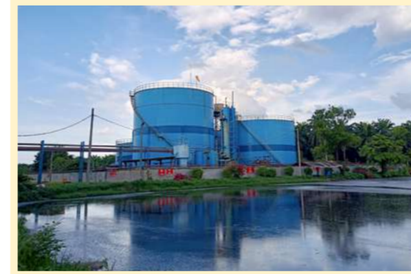
A wastewater treatment plant in one of our units
