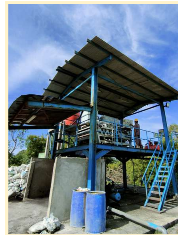
Belt presses are installed in some of our mills to help reduce effluent's COD load
