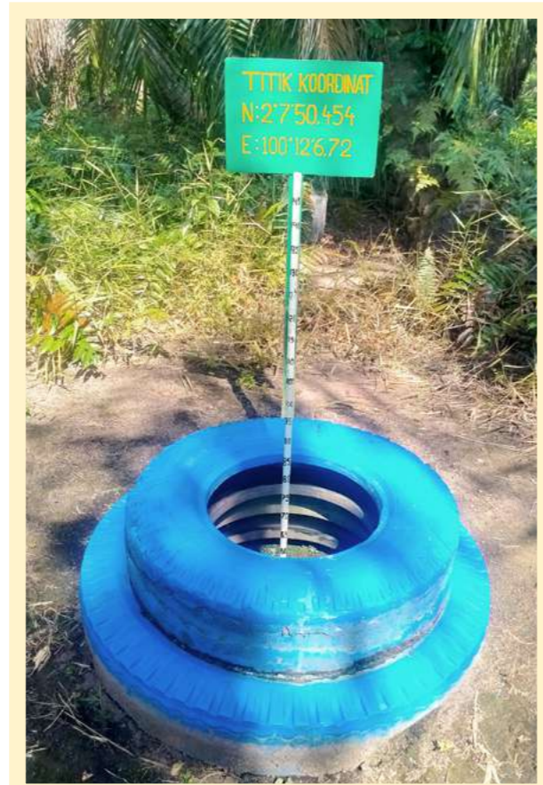
Piezometer is installed to measure and ensure that the water level is maintained at the recommended level
