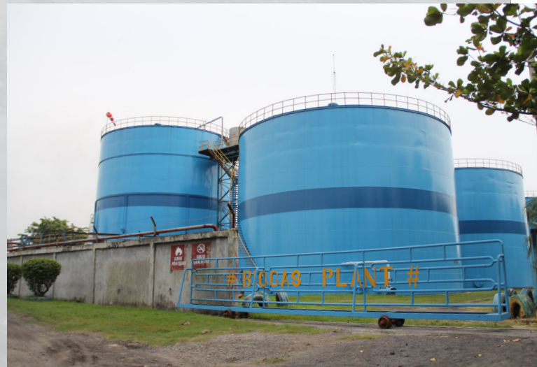
The biogas captured by our methane capture facilities are utilized to generate electricity or bio-hydrogen
